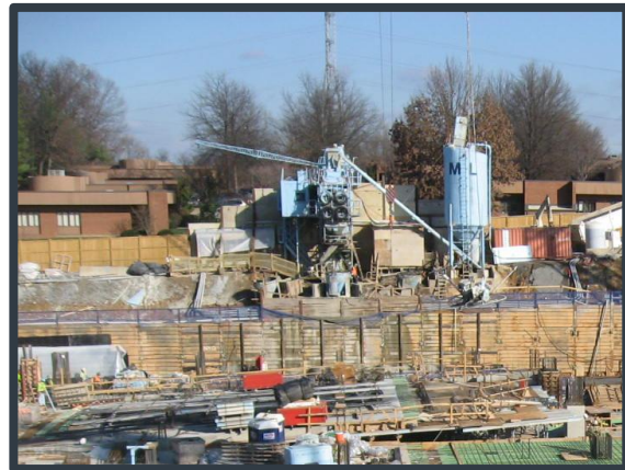
Figure 9: Concrete Batch Plant
